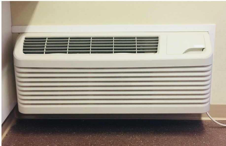
Figure 6 – A PTAC that does not extend all the way to the floor.
